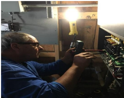
Checking Solar DC Circuit values in the multi string PV inverter for a field of arrays.
