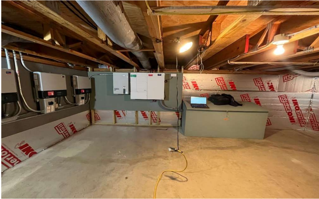
©BPVS 2023: Original SMA Solar Utility Interactive Inverters on left. Six years later a CONEXT XW Battery Based Inverter and Controls at center were added by the homeowner. The laptop in the photo sits on the battery bank cabinet.
