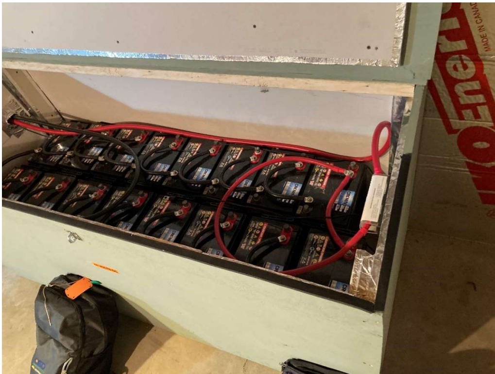
©BPVS 2023: American Made AGM batteries in NEC/NFPA code approved Battery Cabinet. Quality battery banks like this can last 15-20 years in a backup application. For off grid sites, where the solar and battery bank capacity is used every day and night of the year, a battery bank like this can last eight to ten years. BPVS has over 60 installations that rely on batteries.
