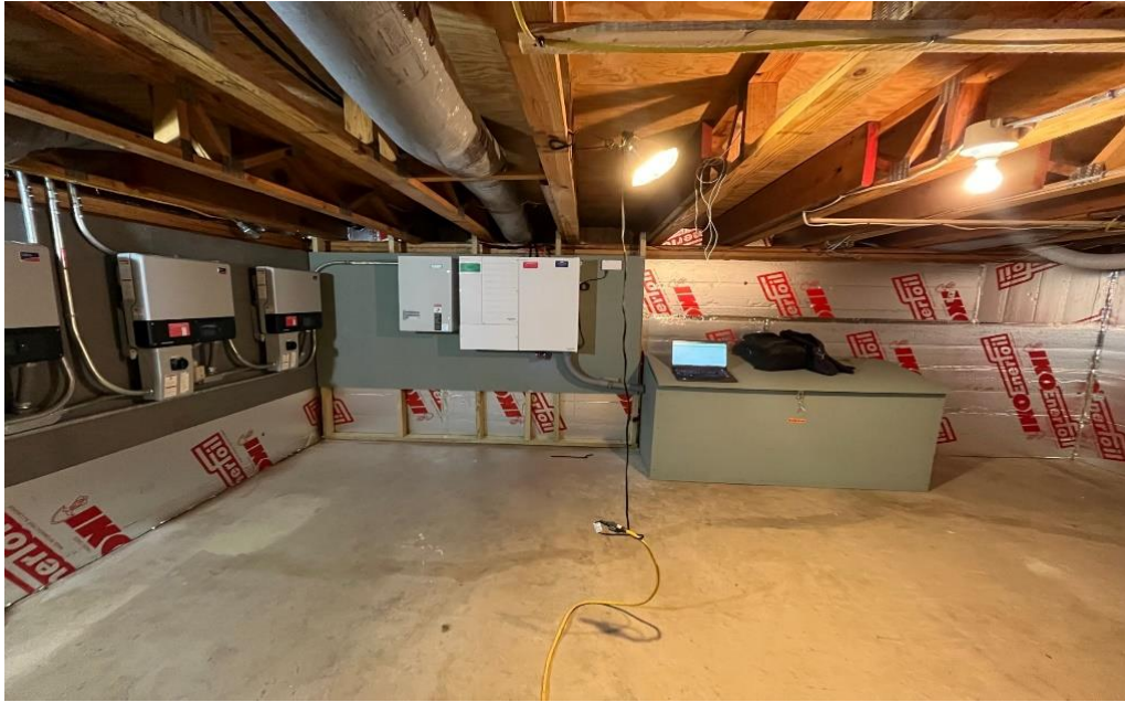
©BPVS 2024: Original SMA Solar Utility Interactive Inverters on left. Six years later a CONEXT XW Battery Based Inverter and Controls at center were added by the homeowner. The laptop in the photo sits on the battery bank cabinet.
