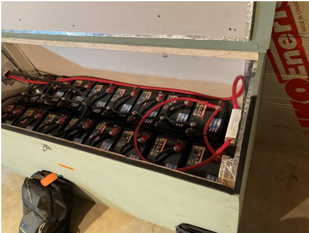
©BPVS 2024: American Made AGM batteries in NEC/NFPA code approved Battery Cabinet. Quality battery banks like this can last 15-20 years in a backup application. For off grid sites, where the solar and battery bank capacity is used every day and night of the year, a battery bank like this can last eight to ten years. BPVS has over 60 installations that rely on batteries.
